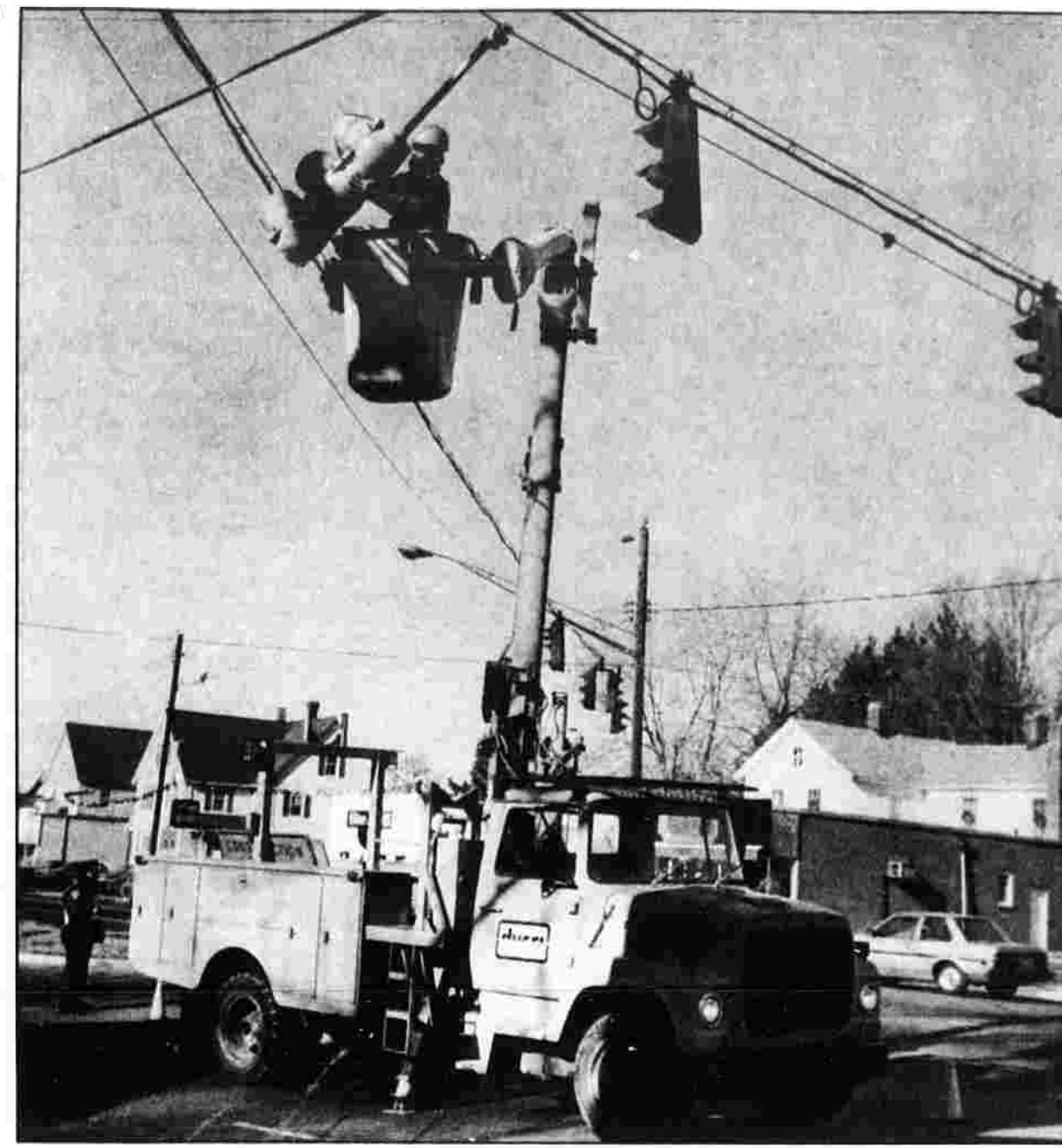
GOING UP — Bob Risley of East Hartford, an employee of Ducel Electrical Contractors in Torrington, replaces a traffic light at the intersection of Center and West Center Streets in Manchester. Various lights across town are being replaced or upgraded.
